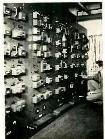
Computer panel where characteristics of the plane are set up contains electronic elements for adding, multiplying and integrating
